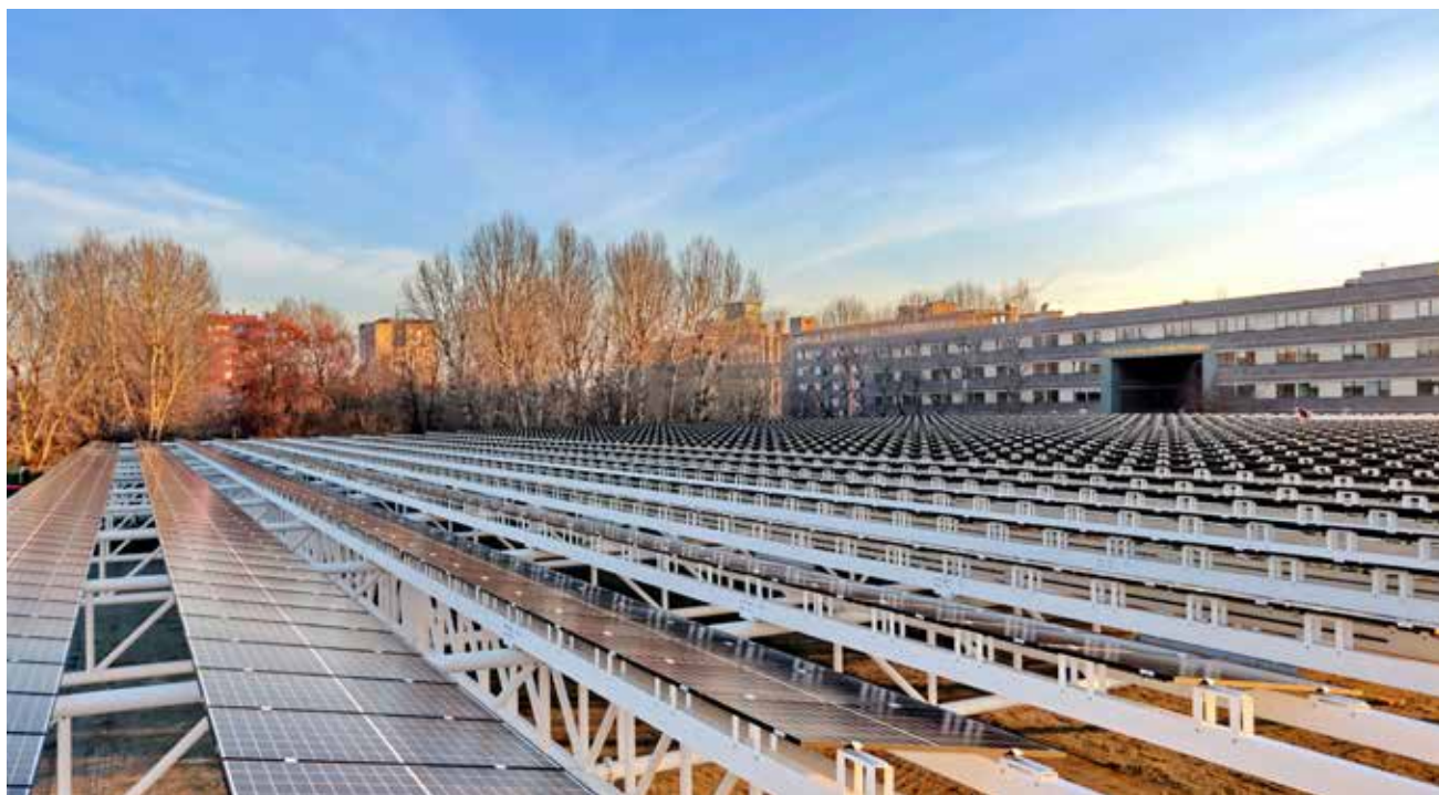
The new new Photovoltaic Park of BPER Banca's Services Centre in Modena
